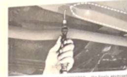
INTERIOR BOX SECTIONS PROTECTED - the fully adjusted TECTYL jet is directed straight forward. Has long range and gives good dispersion.
